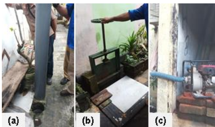
Figure 3. The existing flood resilience system consists of water level indicators at subsurface sewer (a), sluice gates for controlling water level (b), and pumping stations to raise water to the nearest receiving water body (c)
